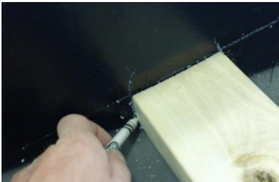
Step 3-3: Place a crossbeam so that its top edge is flush to the line and an outer corner rests on the ground as shown in the illustration above. Hold it in place and trace its outline.
