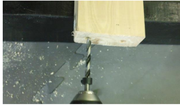
Step 3-6: Make space for the threaded inserts by widening the 13/64" pilot holes already in the crossbeam. Center a 1/4" drill bit on the holes and drill about 1/2" into the crossbeam (W1).
